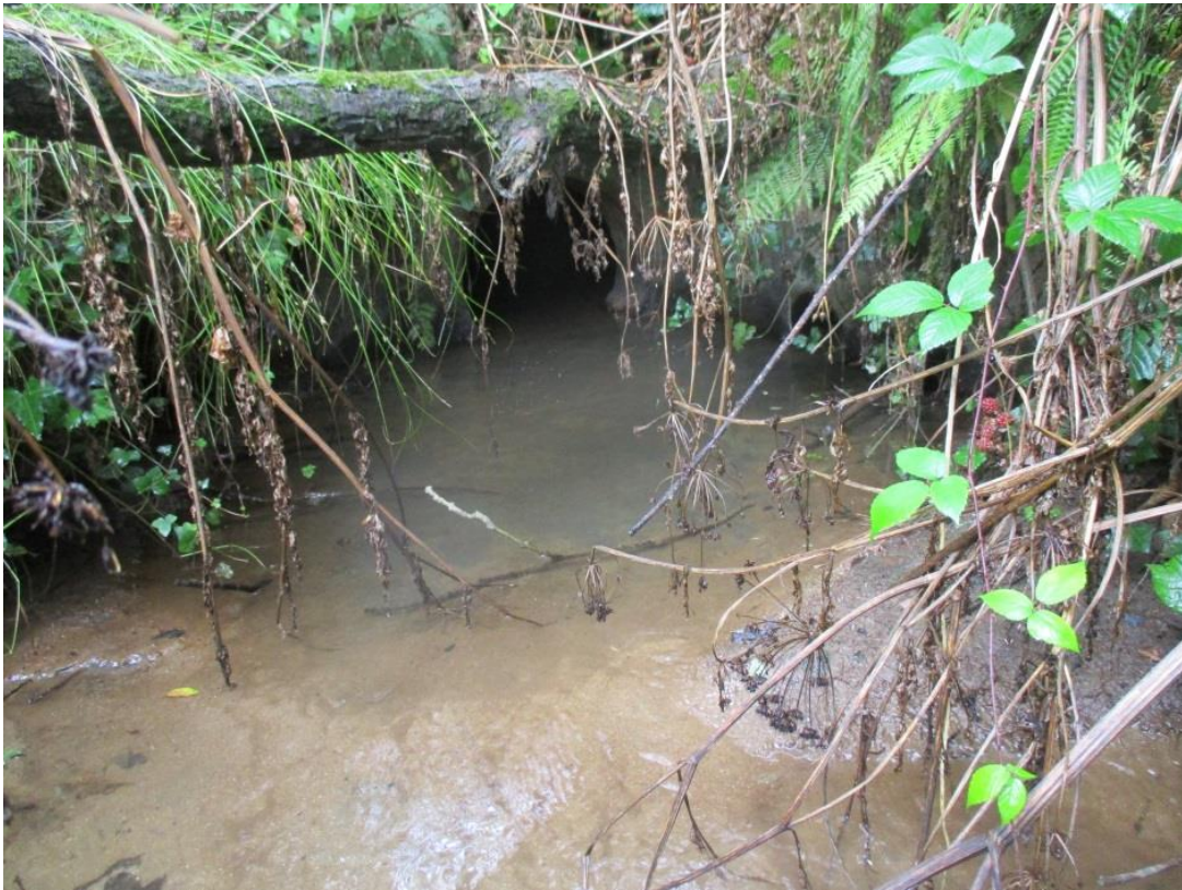
St Austell North sewer storm overflow, 21 st August 2021
